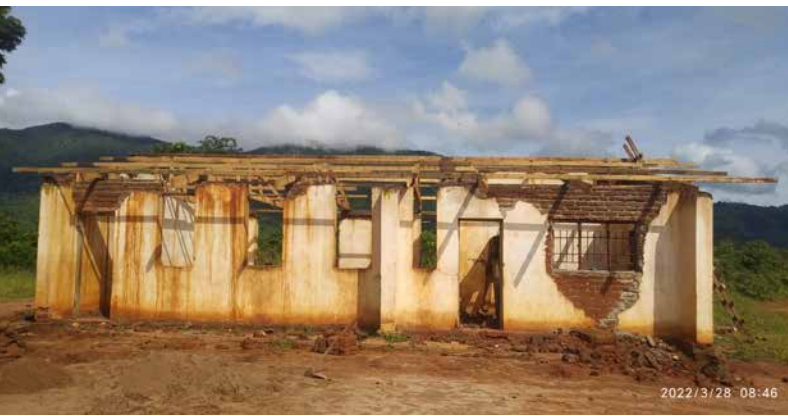
Kapilimuhoto Clinic awaiting new roof
